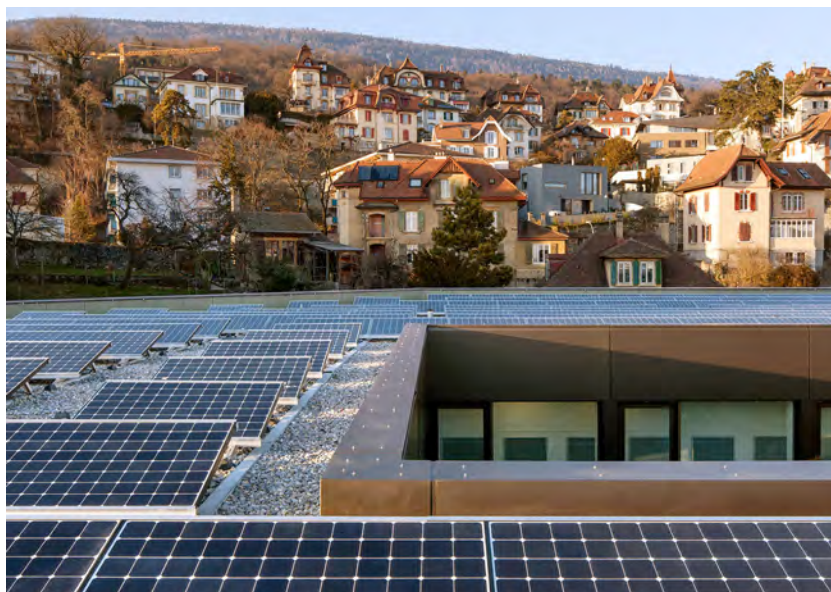
Figure 4. Photovoltaic central on the roof connected to the city's power grid (Picture: Yves André).
